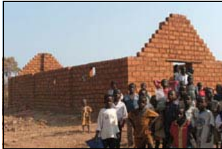
An unfinished Church building. The hope of something big.
