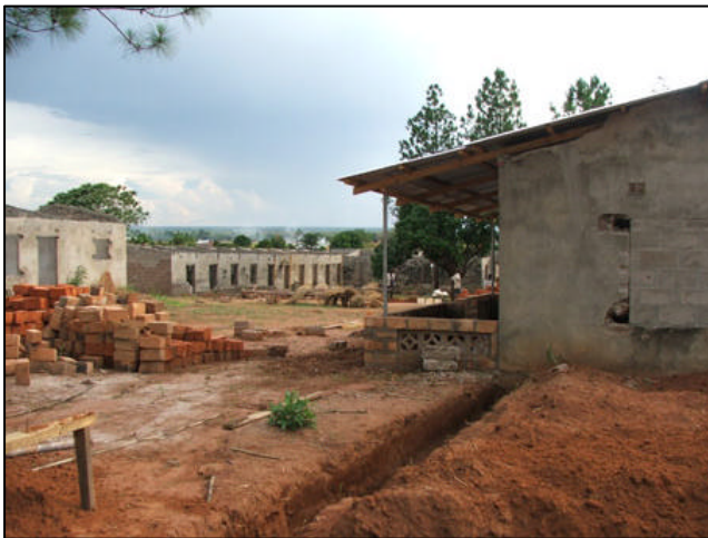
As you can see there is plenty being done and plenty more to do. You can see in the right forefront of the photo our living quarters with the foundation dug for the first ablu-tion block. At the back of the photo is the 'east wing' which is yet to be developed. And on the left of the photo the future dining hall and kitchen building.
