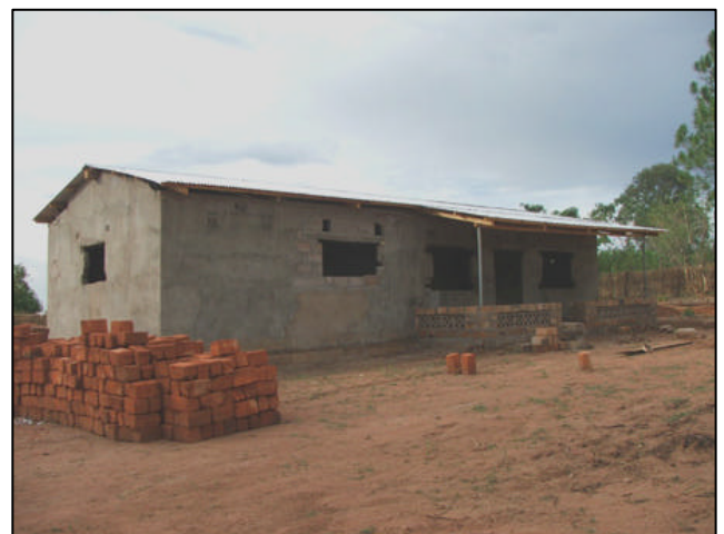
This building will be our living quarters with one bedroom, living room and office. The kids will have small bedrooms in the main building.
